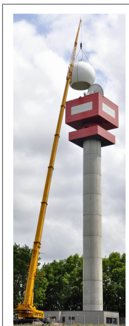
Fig. 2. Installation radar Jabbeke on 13.06.2012
